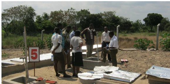
Co-digestion of mixes takes place in dome-digesters underneath the ground
